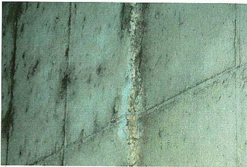
Figure 12: Misalignment in Culvert Exterior Wall
