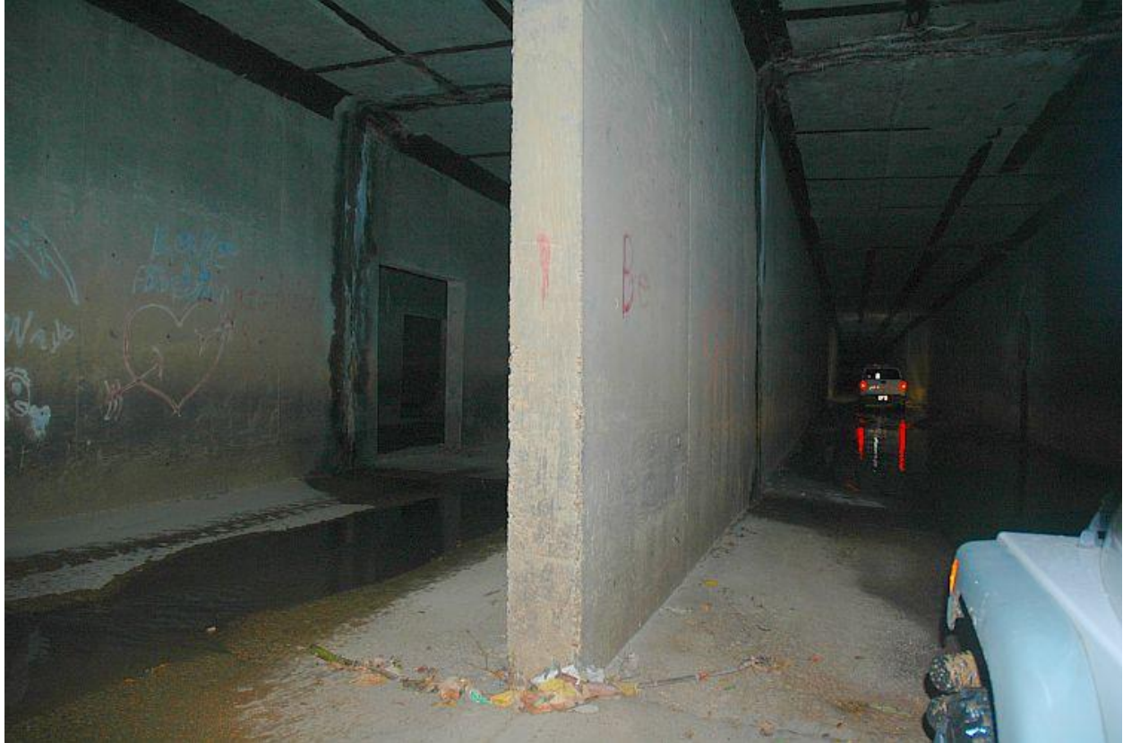
Interior view of Hurricane Creek drainage culvert. There are four individual tunnels.
