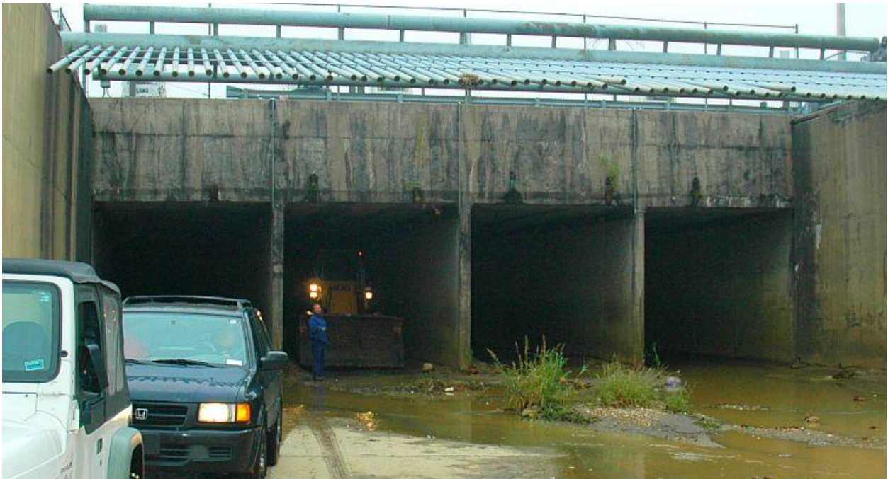
The Hurricane Creek Tunnel which passes beneath Runway 9/27 has 3 interior walls and 2 outer walls. All five are badly fractured directly beneath the runway.
