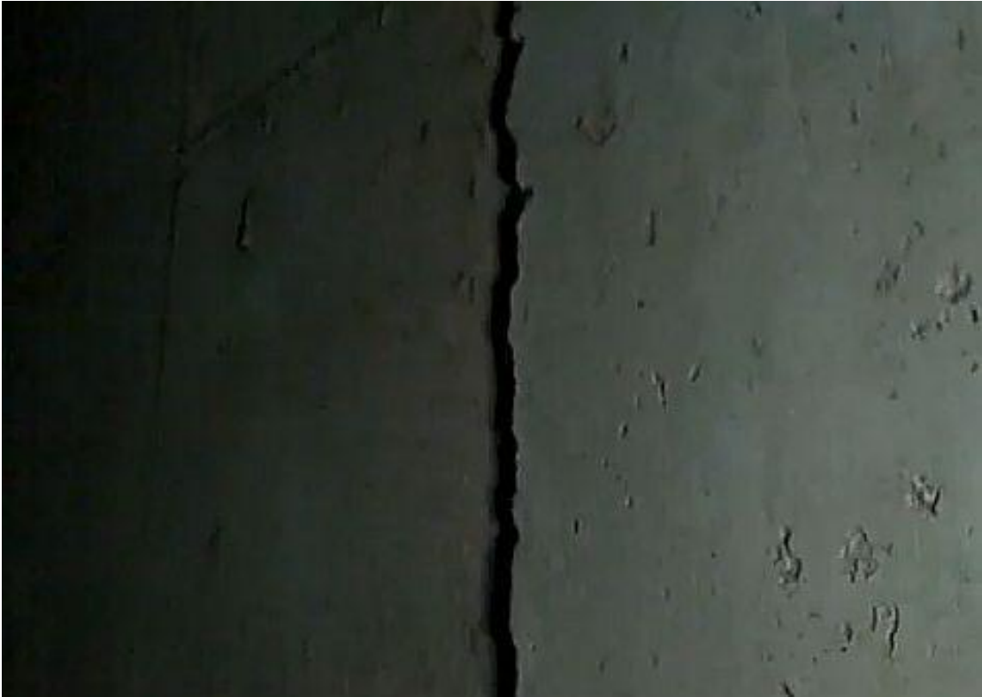
These are video images of the damaged walls holding up the runway at Memphis International
