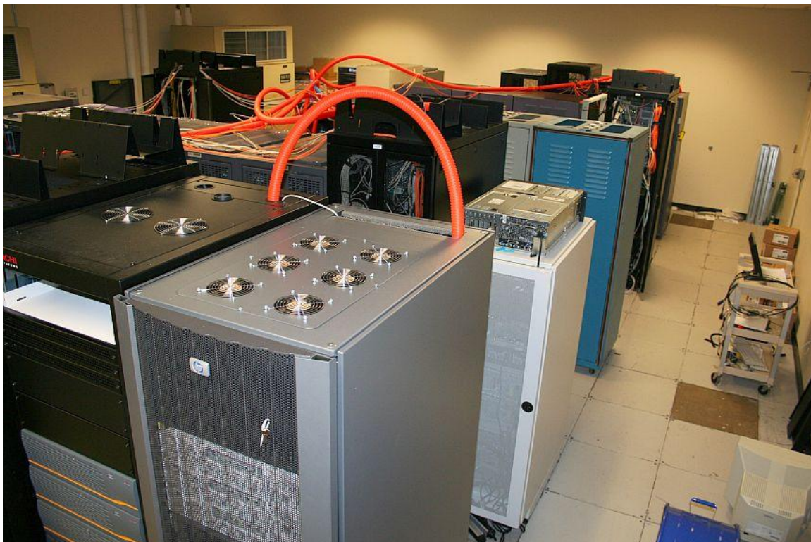
WHQ Building D 2 nd Floor Computer Room
