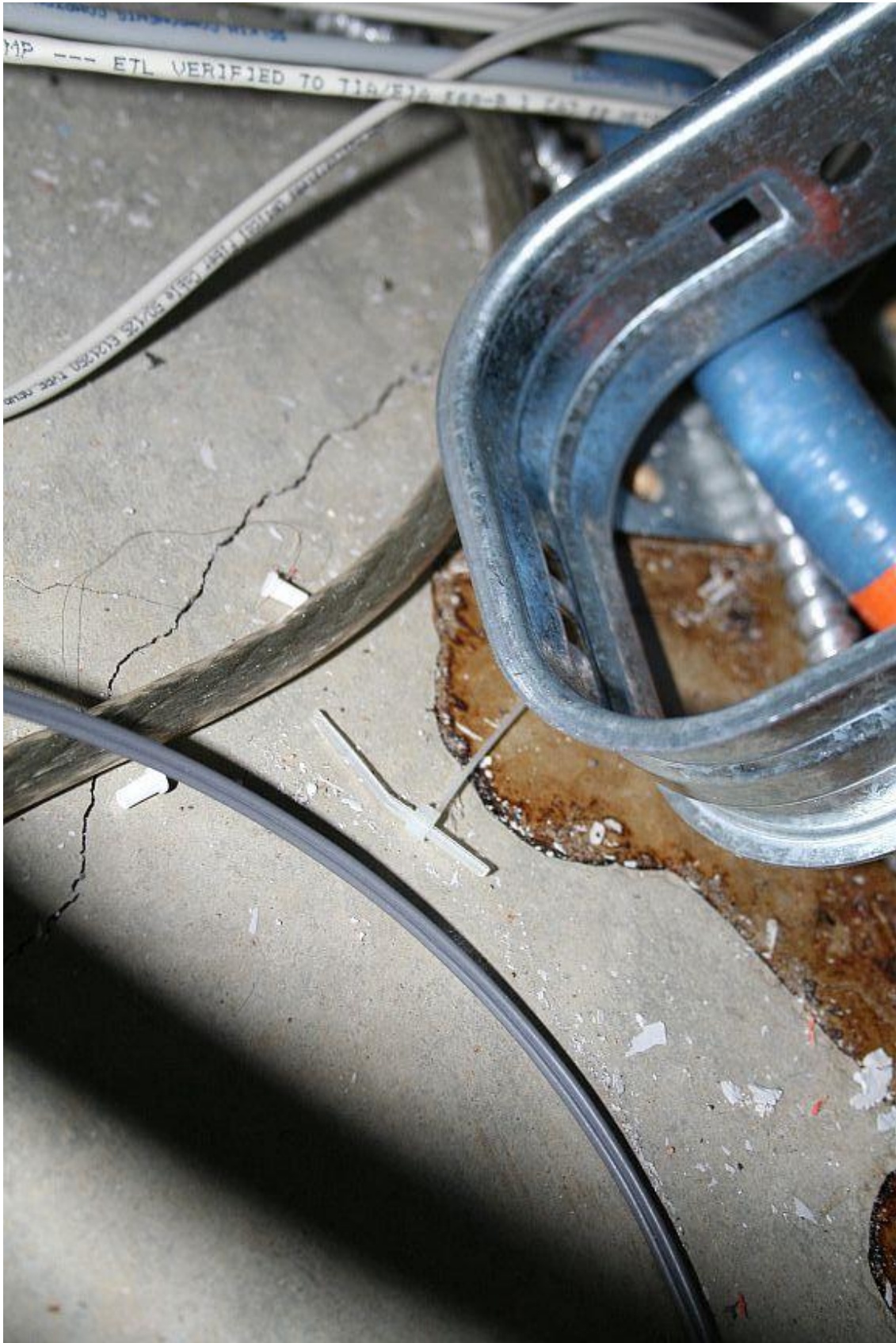
Floor Crack at Upper Left
